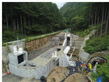
Seinaiji hydro power (current status)
